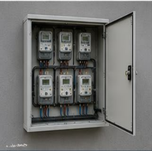
WALL MOUNTED METER PANEL
