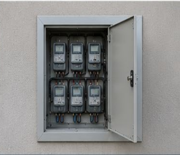
RECESSED METER PANEL
