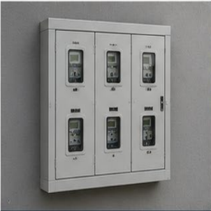
SURFACE MOUNTED METER PANEL
