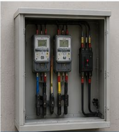
CT METERING PANEL
