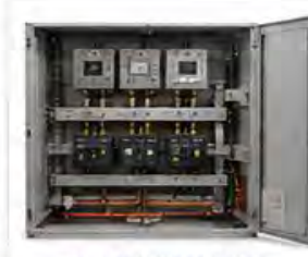
SYNCHRONIZATION & CHANGEOVER PANELS Seamless power transfer and system reliability.
